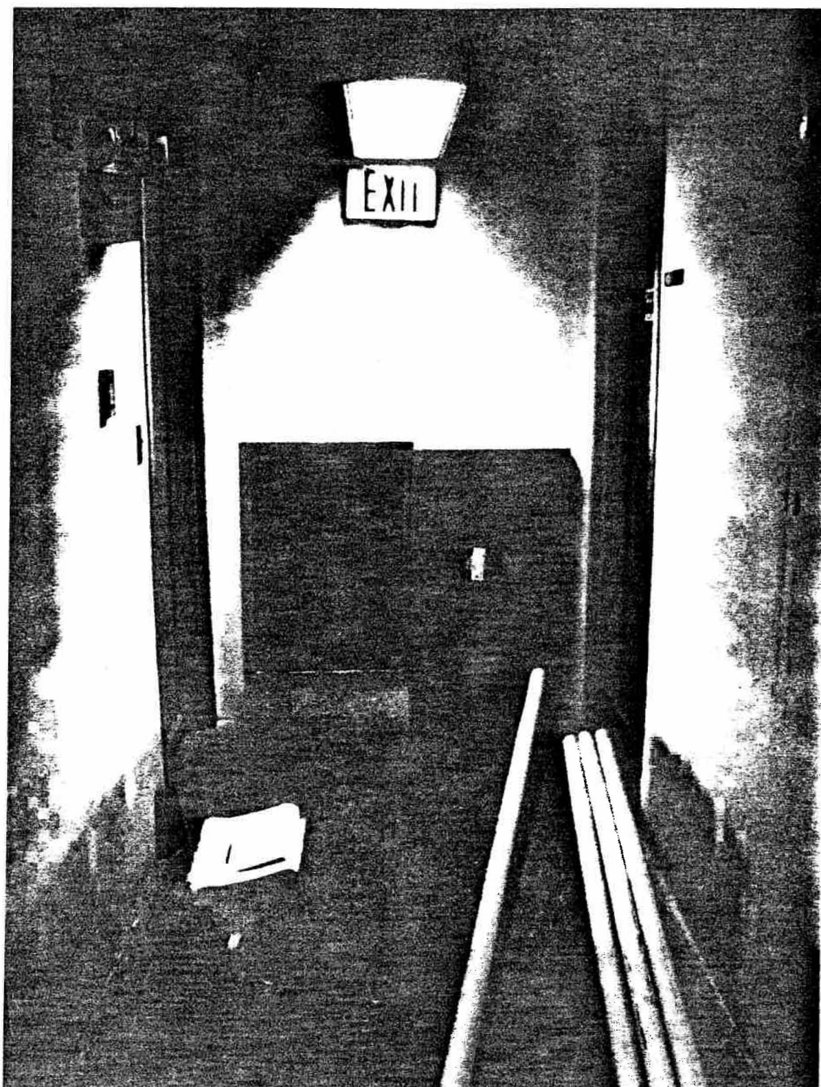
Photo 4.2.13-1 Fourth Floor Elevator Vestibule – Uninsulated Access Door
