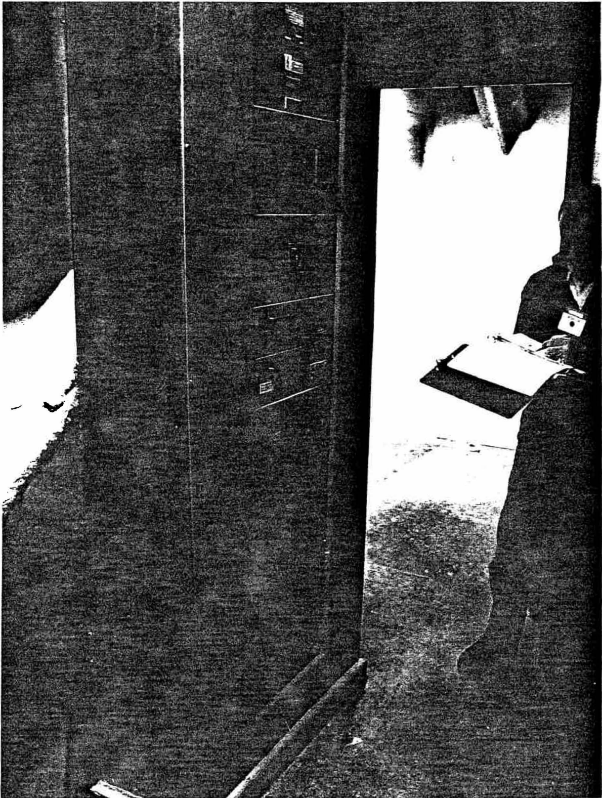
Photo 4.2.8-4 Electrical Equipment in Room #927A
