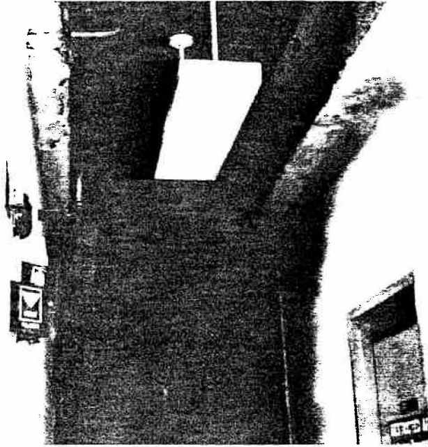
Photo 4.2.9-1 Door to Room 828 on Right – No Rated Wall above Beam Above Door
