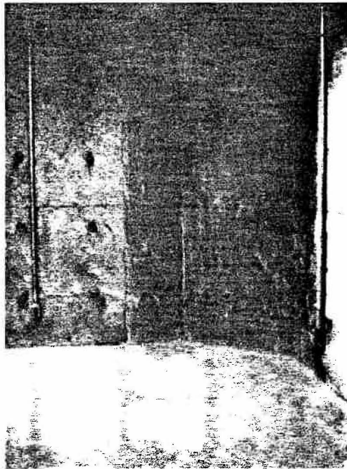
Photo 4.2.9-2 Exterior Wall in Room #828 – Moisture at Horizontal Joint
